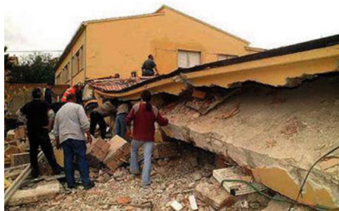
Fig. 14.14 Francesco Jovine school of San Giuliano di Puglia, after its collapse during the 2002 Molise & Puglia earthquake ( M = 5.9 )
