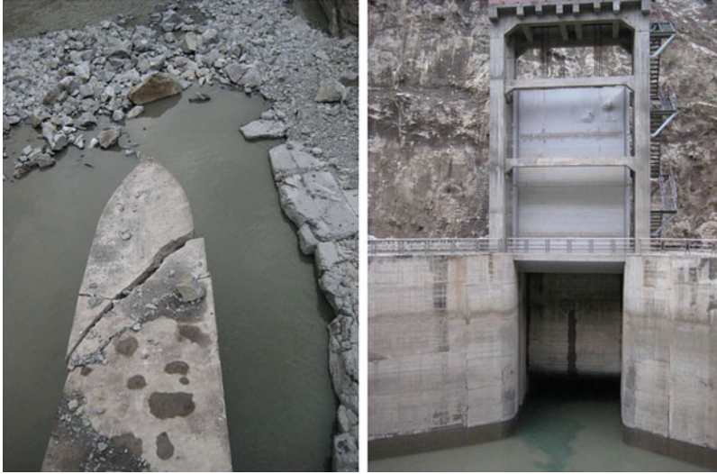
Fig. 20.5 Damaged pier of Futan weir looking downstream ( left ) and damage of sliding gate for power intake (indentation of steel leaf from rockfall) ( right ) caused by the 2008 Wenchuan earthquake in China
