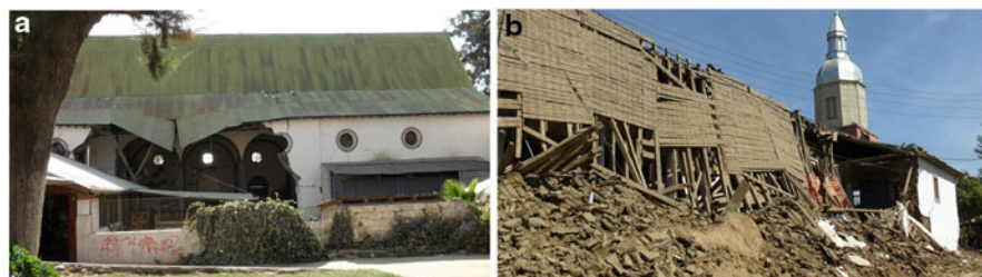
Fig. 15.1 (a) Church in Lalol, Colchagua, Chile. Collapse of the lateral adobe wall, strengthened by shotcrete. (b) Church in Curepto, Maule, Chile. Collapse of the lateral adobe wall, strengthened by shotcrete
