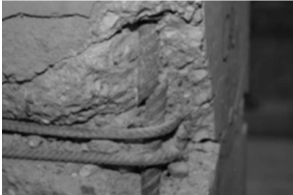
Fig. 4.15 The mistake in the construction of the hoops (and the resulting impaired confinement) led to heavy damage of the precast column in the PRECAST full-scale test
