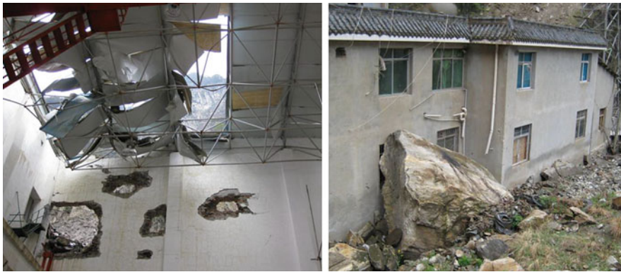
Fig. 20.4 Infill wall and roof of powerhouse punctured by high-velocity rocks ( left ) and wall damage of building of Shapai power plant by large rock ( right ) caused by 2008 Wenchuan earthquake
