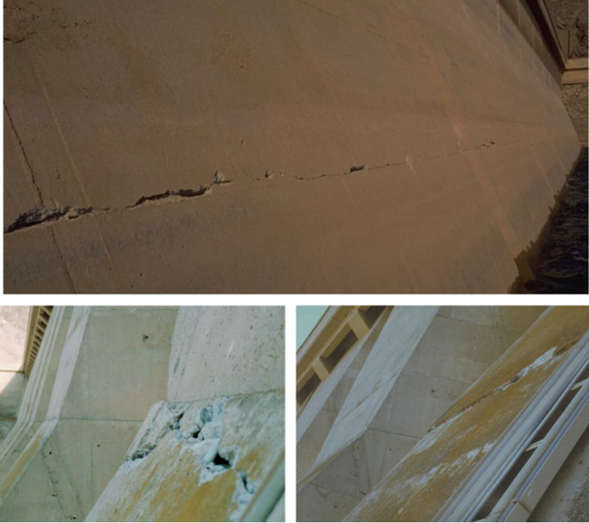
Fig. 20.1 Crack at upstream face ( top ) and at the kink ( left bottom ) and crack showing sliding movement of wedge formed by cracks at the kink ( right bottom ) of the buttress at the downstream face of the Sefid Rud buttress dam caused by ground shaking during the 1990 Manjil earthquake in Iran
