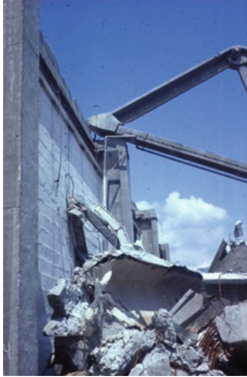
Fig. 4.9 Collapse of the roof structure in Montenegro earthquake due to soil effects and poor connections
