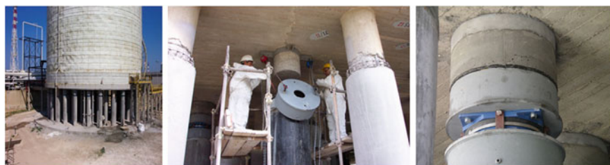
Fig. 14.16 One of the three tanks of the Company Polimeri Europa of the Italian ENI Group located in Priolo, which were seismically retrofitted using U.S. FPS devices in the years 2005–2008 and one of the isolators during and after its installation. To the knowledge of the authors, this is the only application of SI to chemical plants and components so far existing in Italy (prior to the 2009 Abruzzo earthquake, it was also the only application of CSS devices in Italy)
