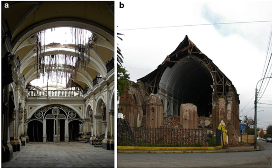
Fig. 15.2 (a) Ica cathedral, (Peru) collapse of the timber barrel vaults. (b) Collapse of the brickwork façade of the Church San Francisco of Curico, revealing the timber structure supporting the roof. Maule, Chile
