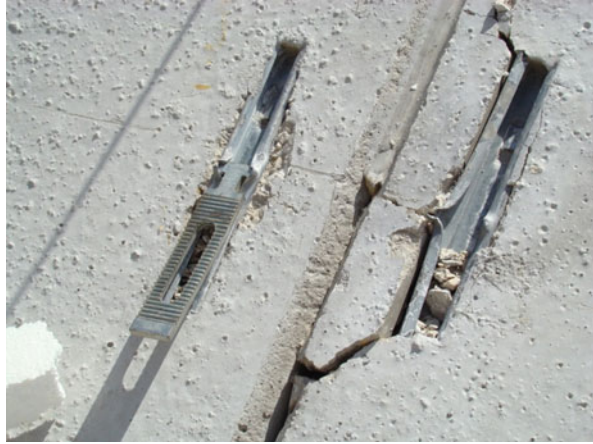
Fig. 4.23 Failure of the traditional hammer-head connection during the Emilia earthquake
